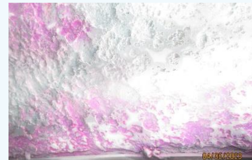
Leak from deep pits
