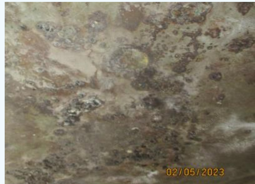
Cleaning showed high corrosion to old SS 304 plate; And pitting attack in the DSS plate
