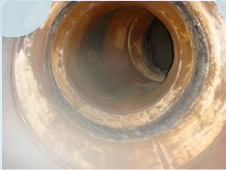
ENBBI, SAFANIYA WATER DISPSAL SYSTEM UPGRADE
