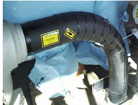
A flowline showing an M2 fitted to the inner bend radius
