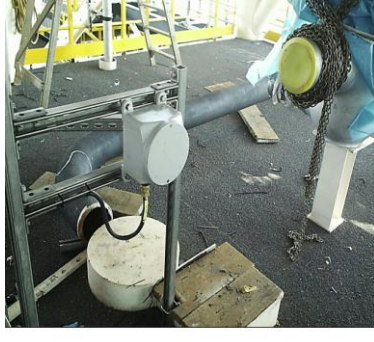
A small hazardous area enclosure for connecting the M2 to extension cables
